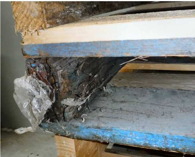
Figure 4: Stringer at left deeply split despite nail plate over split. Plate is damaged in use and has wrapping caught on exposed sharp edge. Spider webbing, dead millipedes, food dust and surface mould also present.
