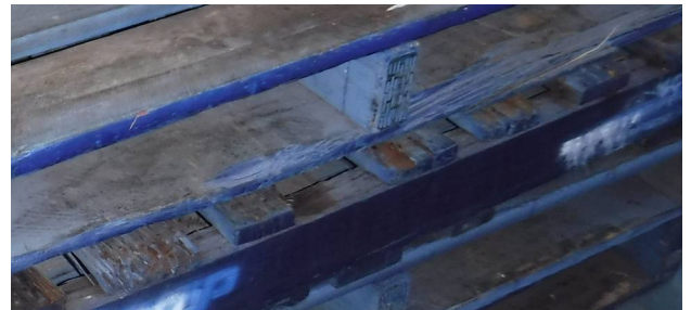
Figure 5: Disintegrating deck boards with protruding nails, splinters, and signs of timber decay.
